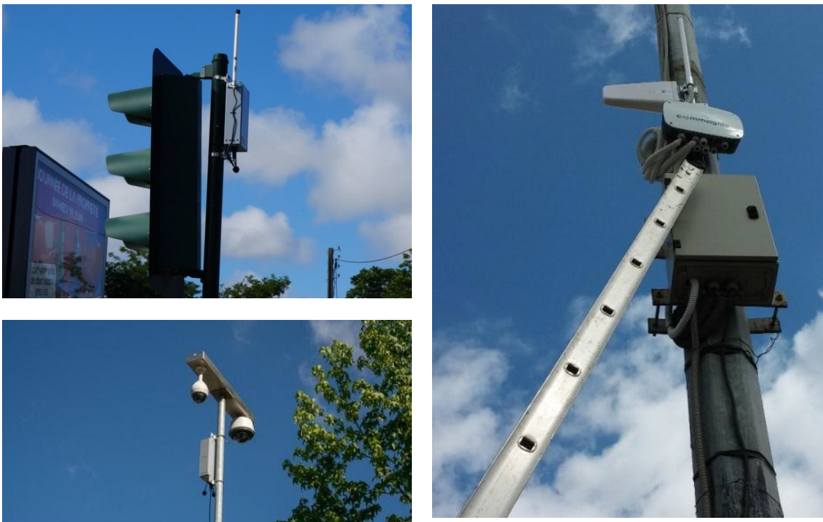
Figure 13: Connected Roads Infrastructure: Top-left: router and WiFi antenna, Right: Router, the external 3G antenna and stick antenna, Bottom-left: Roadside monitoring unit
