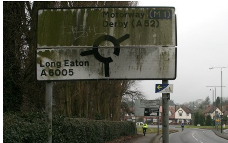
Figure 17: Example of a poorly maintained road sign that may be difficult for CAVs to interpret [Source: http://s0.geograph.org.uk/geophotos/01/66/92/1669239_d416144e.jpg ]
