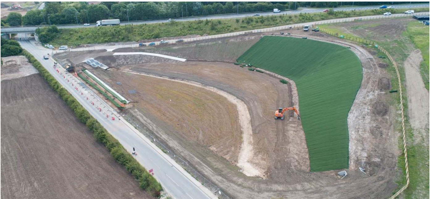
A lagoon under construction as part of the Cottingham and Orchard Park Flood Alleviation Scheme
