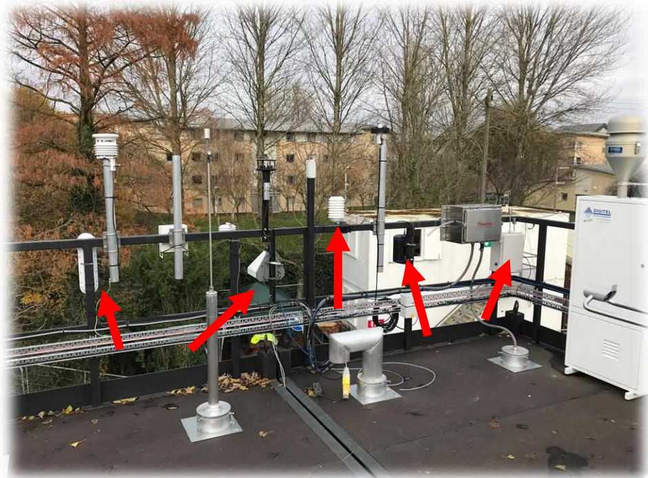
Manchester site, full installation
